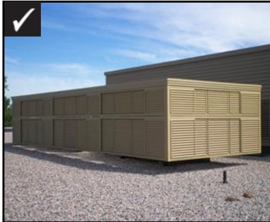
Screened Roof-top Equipment
