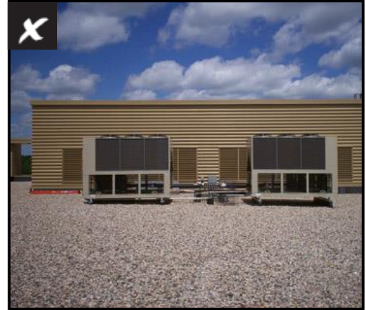
Unscreened Roof-top Equipment
