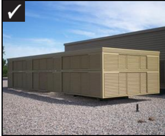
Screened Roof-top Equipment
