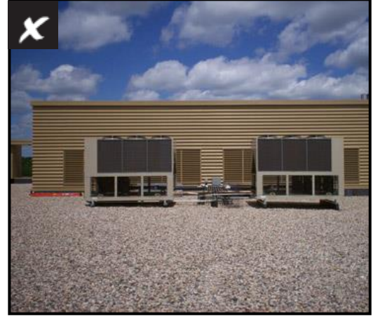
Unscreened Roof-top Equipment
